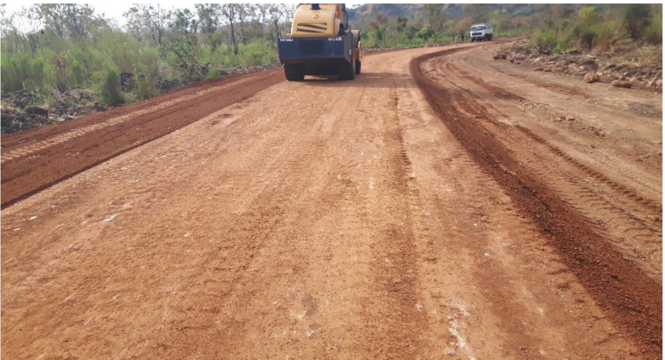
Gravel road construction for south Sudanese refugee in Nguyyiel refugee camp, Gambella (UNHCR support)
