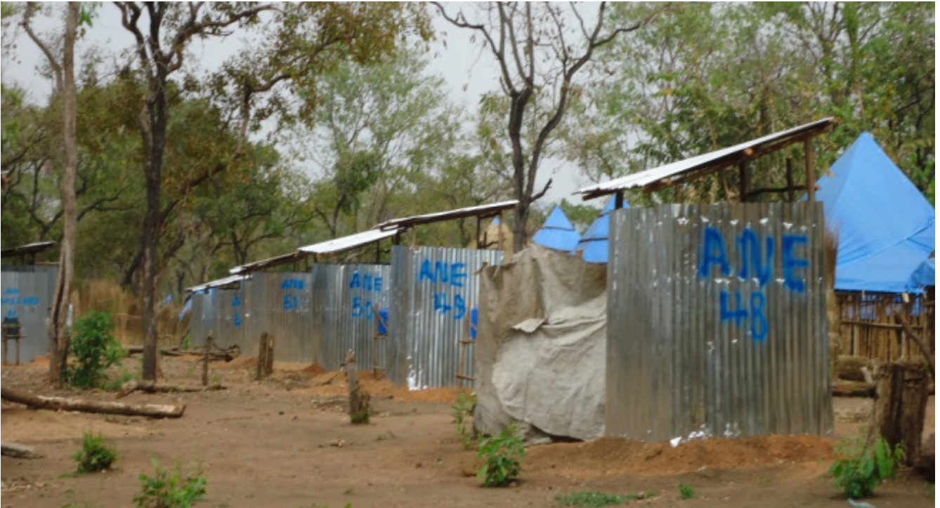
Construction of family latrine for south Sudanese refugee in Jewi refugee camp, Gambella (UNHCR Support)
