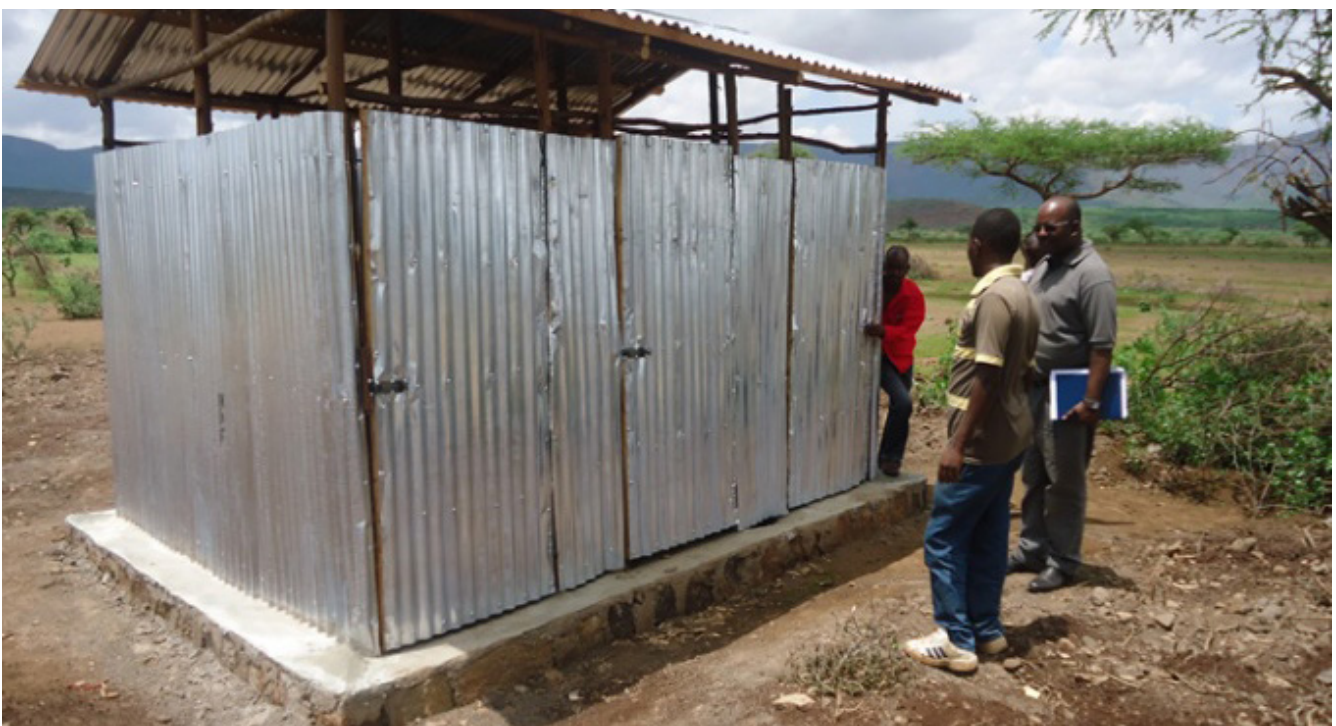
Construction of family latrine for south Sudanese refugee in Jewi refugee camp, Gambella (UNHCR Support)
