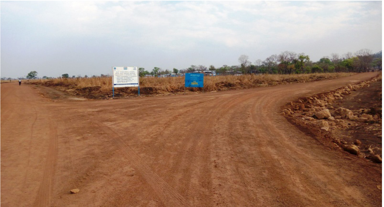
Gravel road construction for south Sudanese refugees in Nguyyiel refugee camp, Gambella (UNHCR support)
